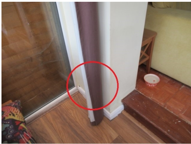
9. Wall staining in the dining room
