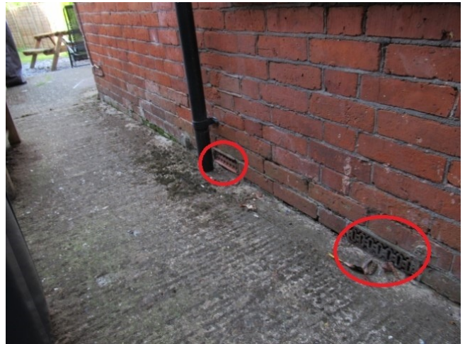
4. External face of area where damp detected
