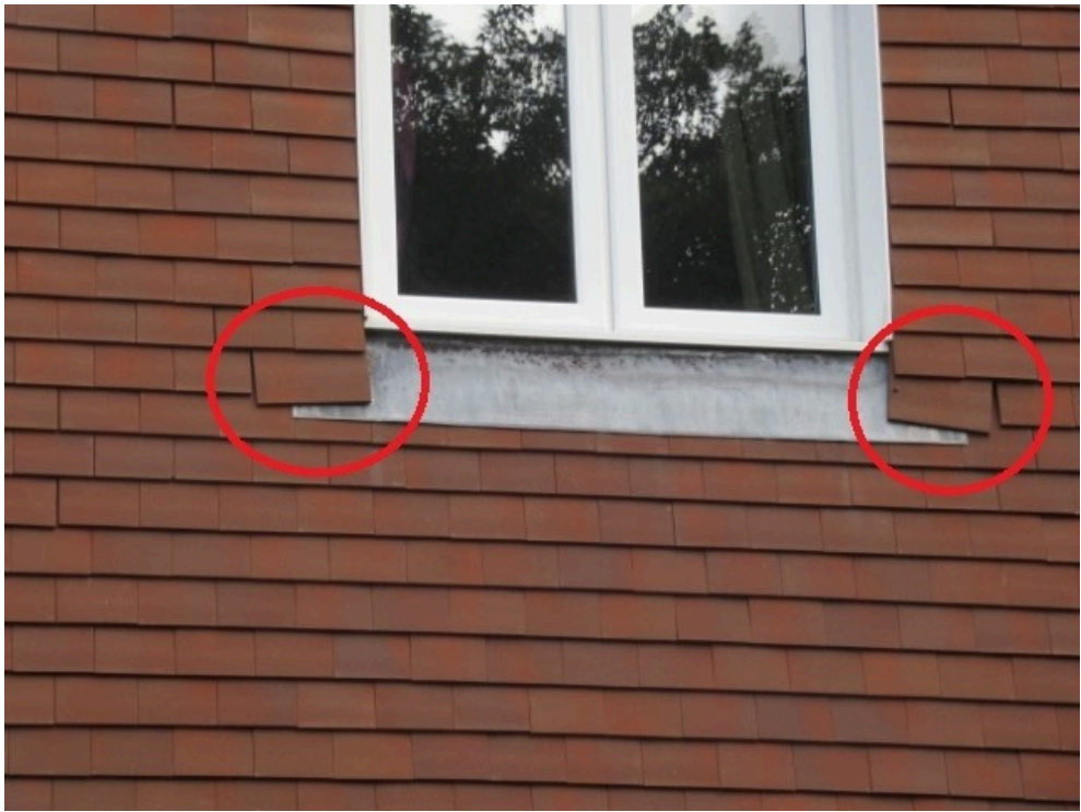
Misaligned tiles at the front
