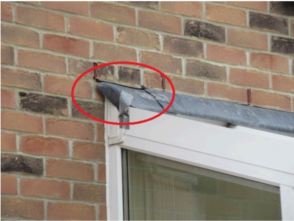
Loose and taped flashing for the living room extension roof at the back
