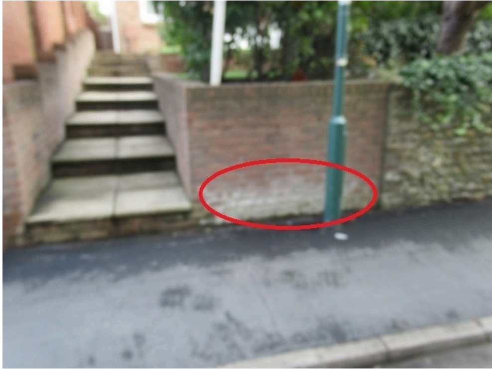
Retaining front wall has no visible drainage outlets
