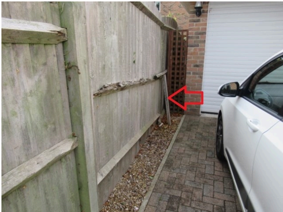
Fence adjacent to the garage is propped and worn
