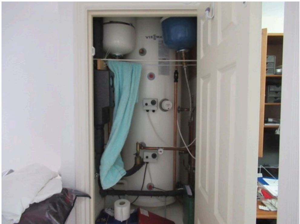
Hot water storage cylinder
