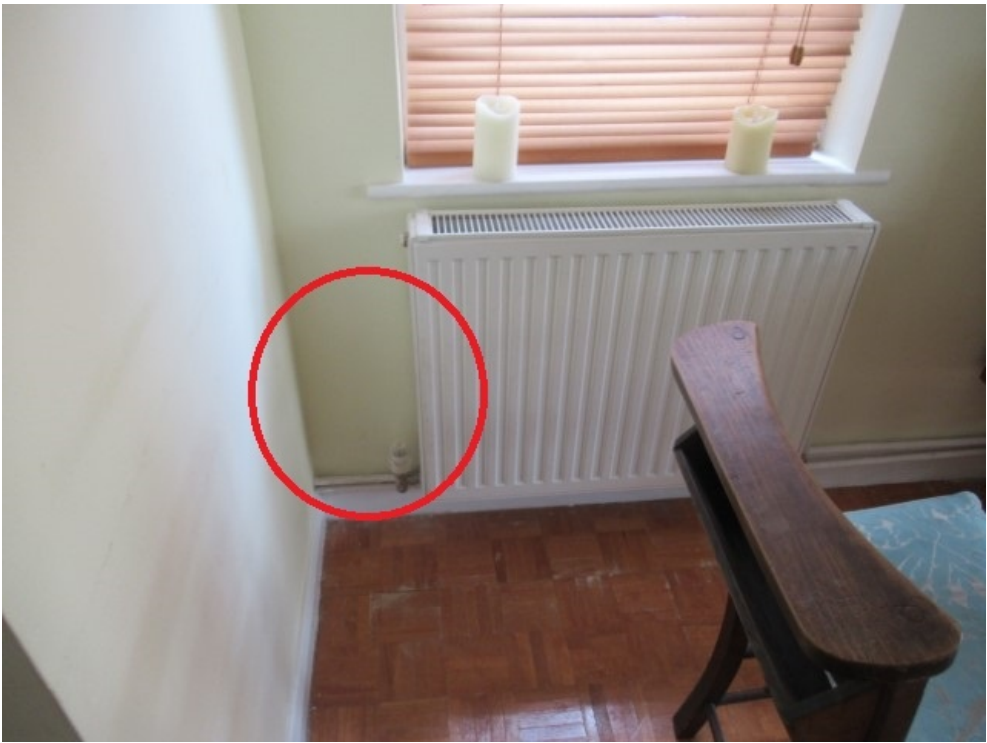
Area of dampness in the living room
