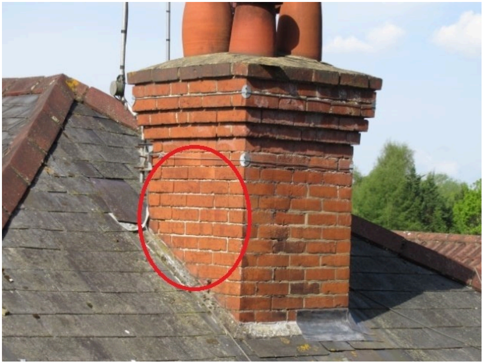
Worn pointing on the left side
