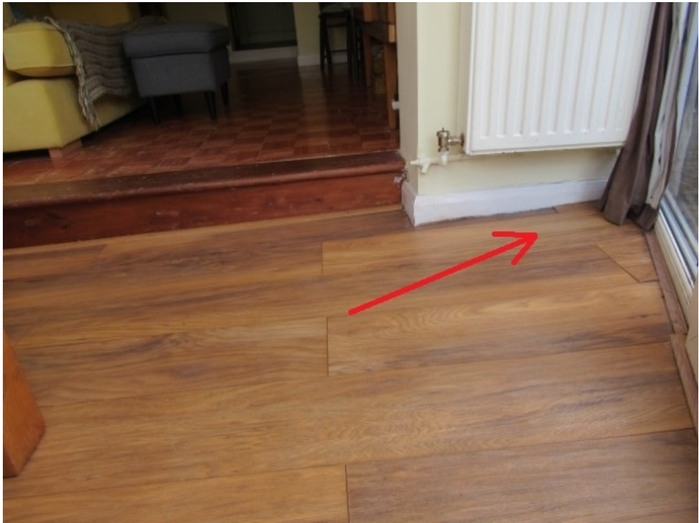
Floor slopes up to the junction with the house
