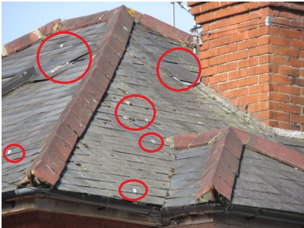
Slipped slates and tingles on the front and left side pitches
