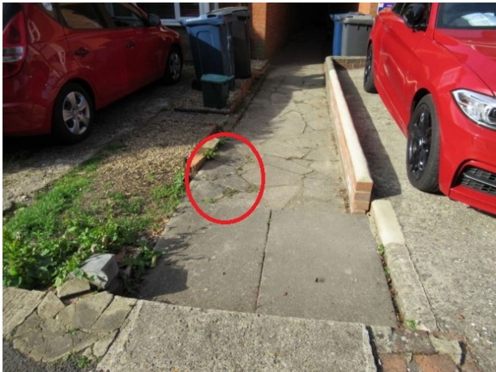
Uneven paving on the shared path at the front
