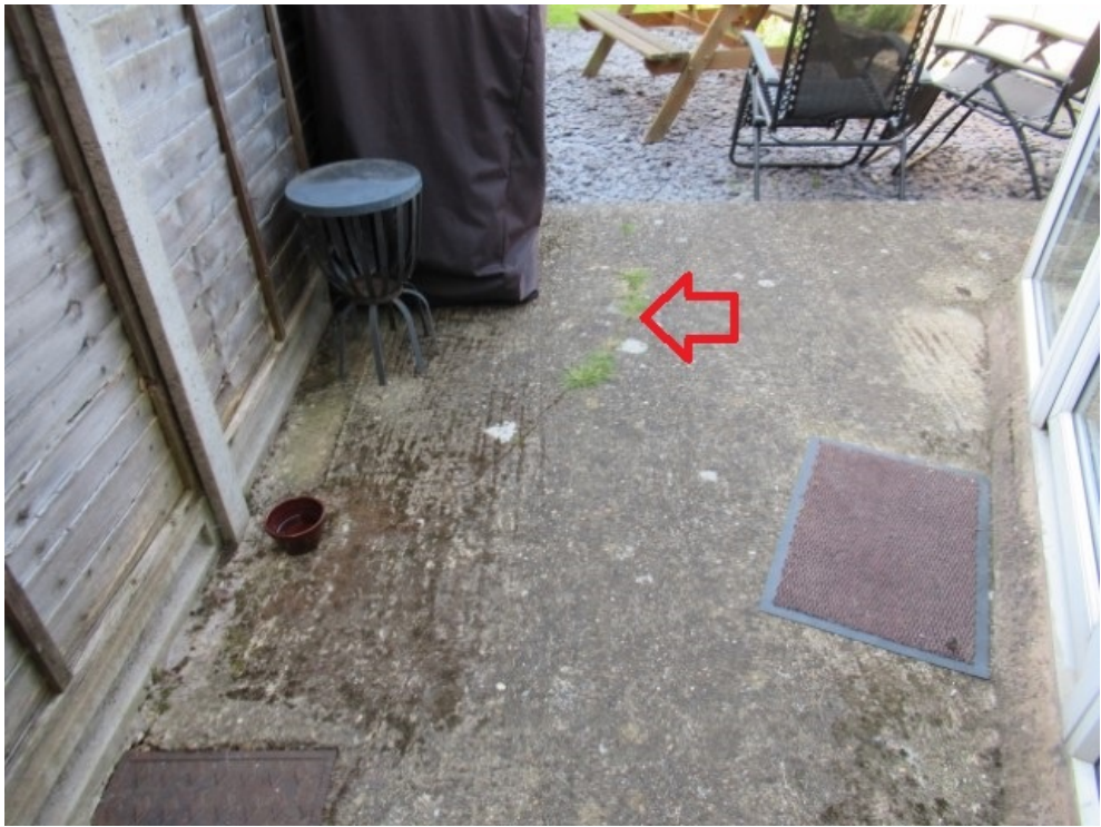
Settlement cracking of the rear patio
