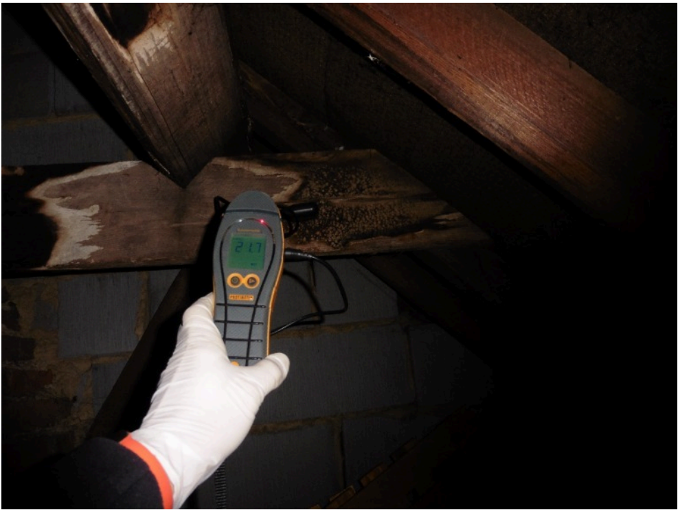
Normal moisture readings recorded
