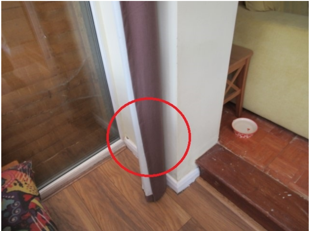
Area of dampness
