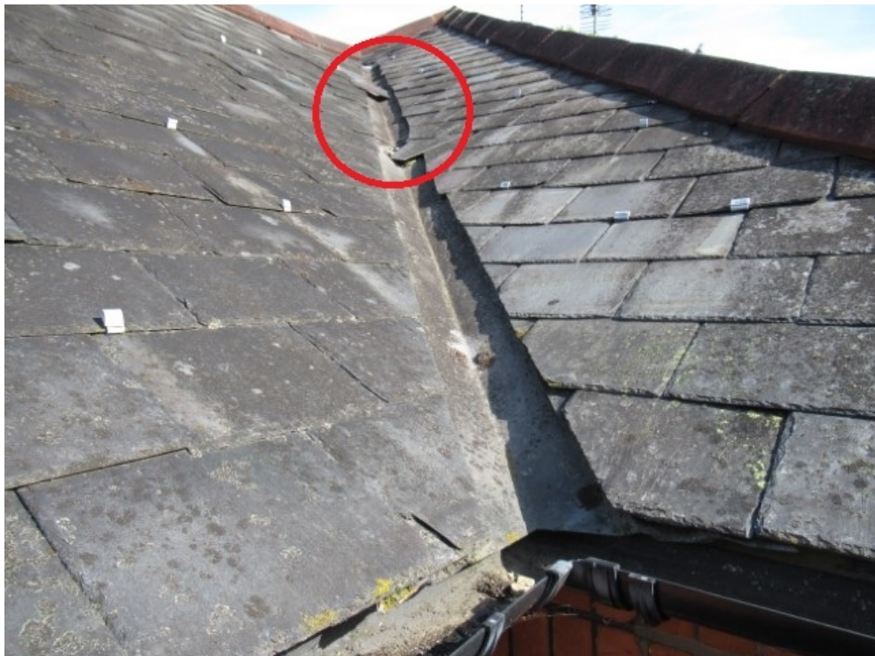
Slipped slates in the rear valley
