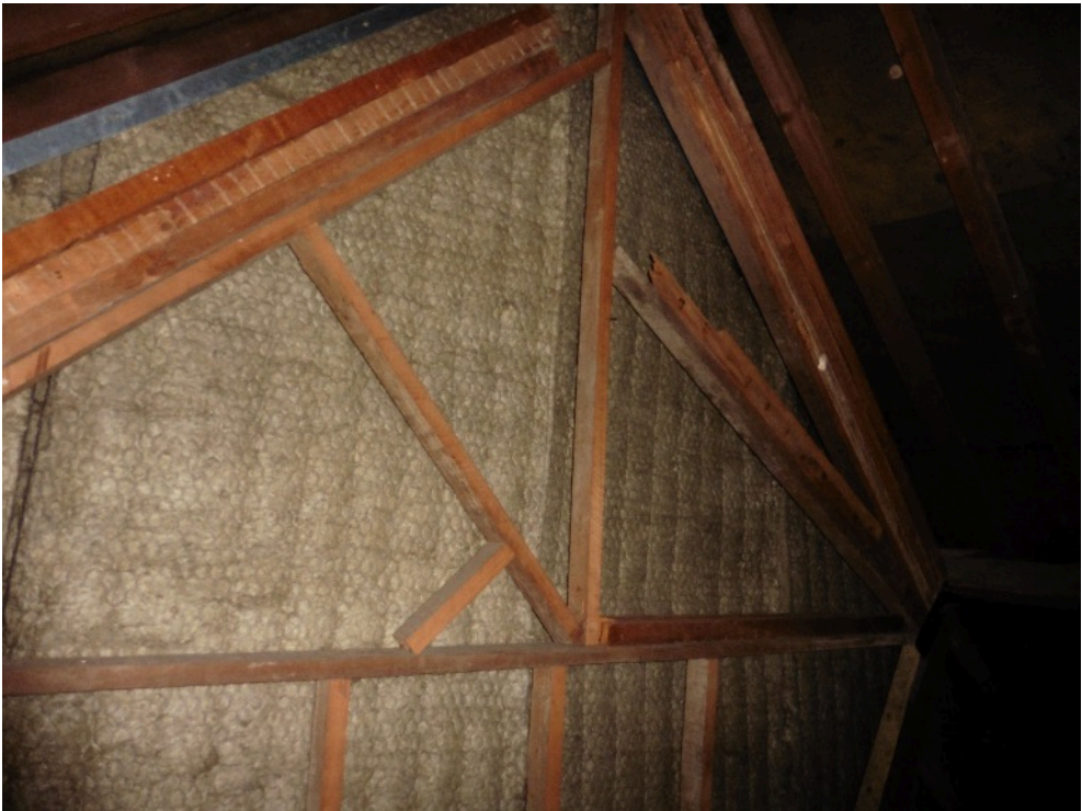
Fibrous material forming fire wall
