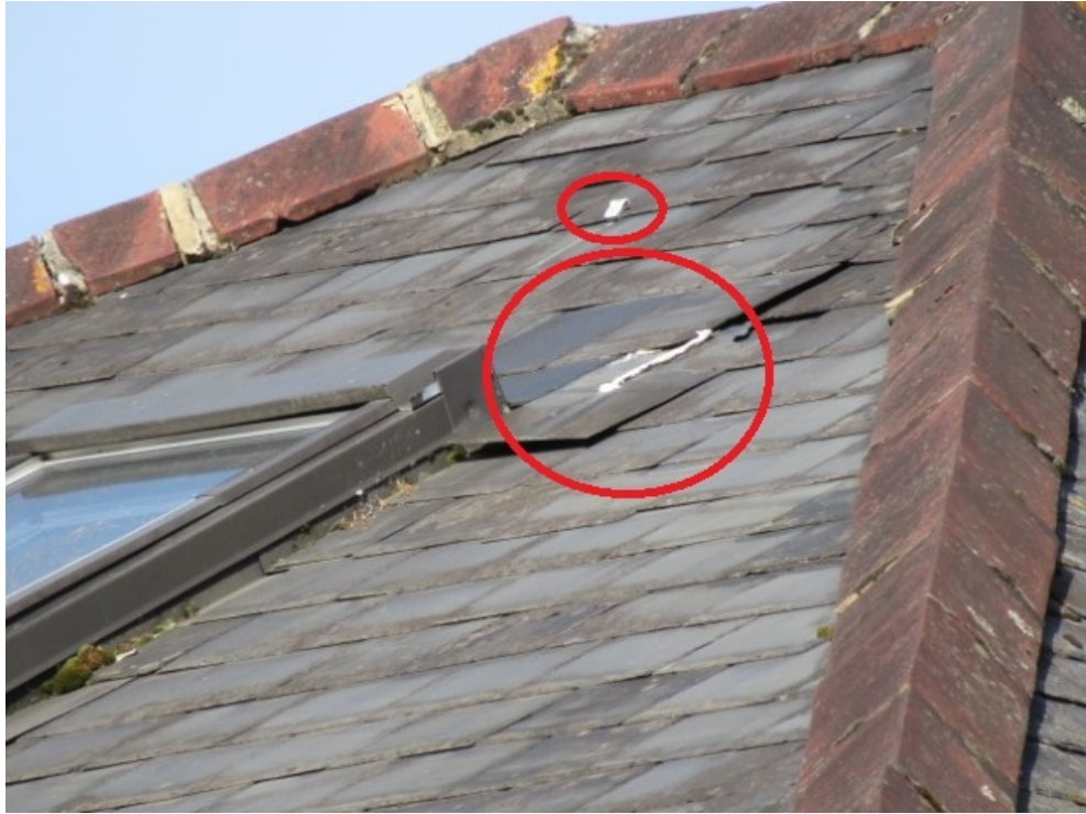
Slipped slates and tingle on the left side pitch
