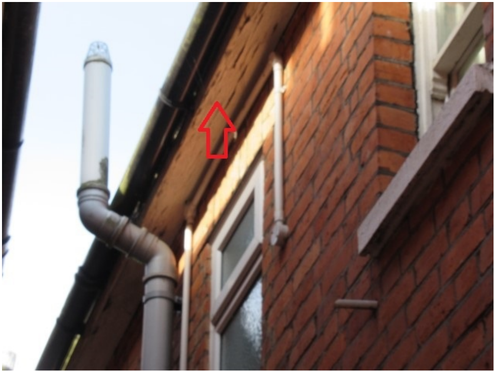
Poorly maintained soffit on the left side
