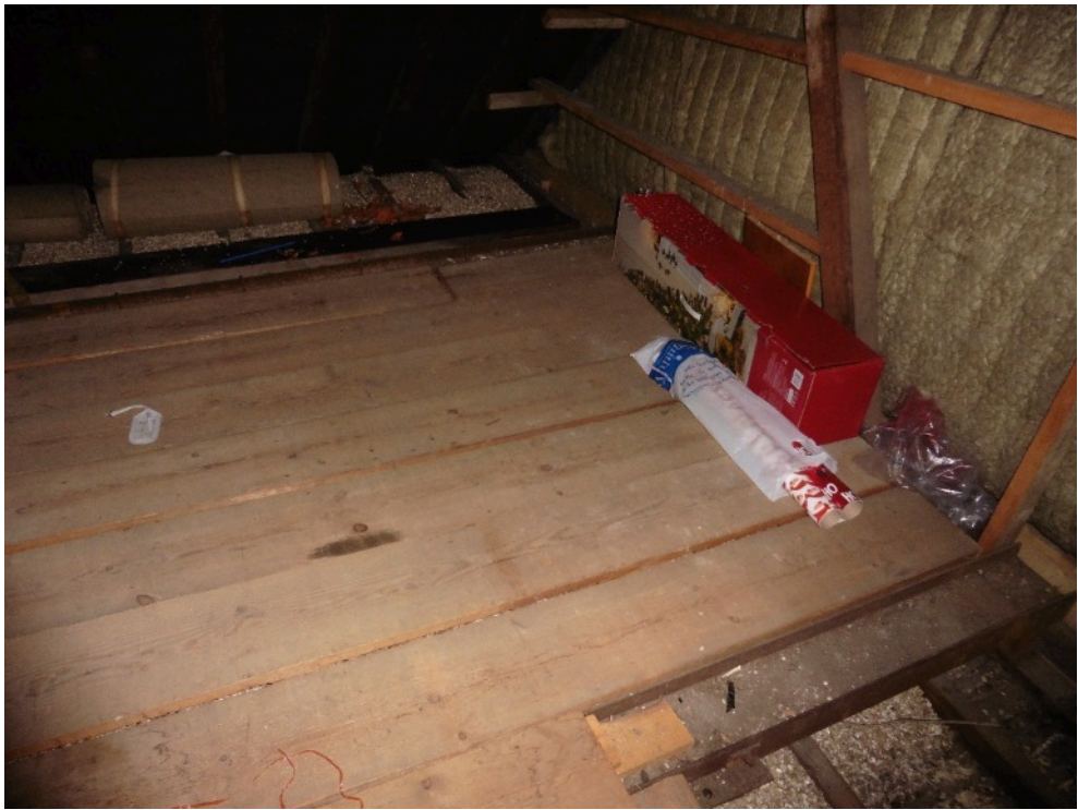
Loose floor boards
